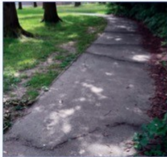
A Wingerworth footpath awaiting repairs
